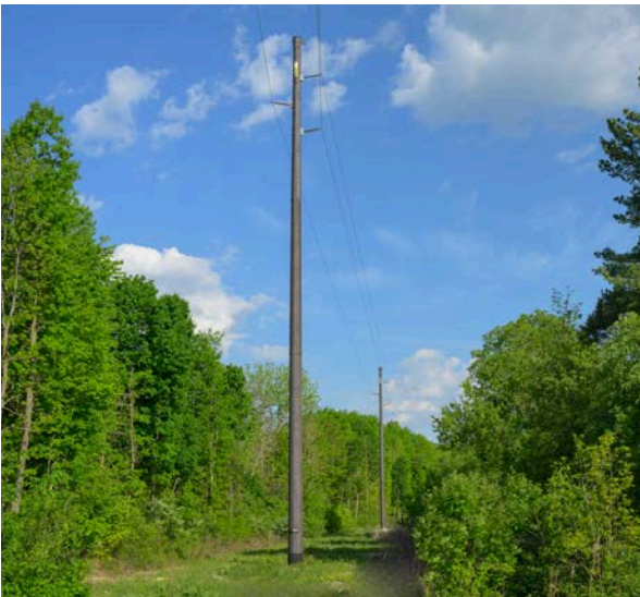
Natina-treated utility poles
