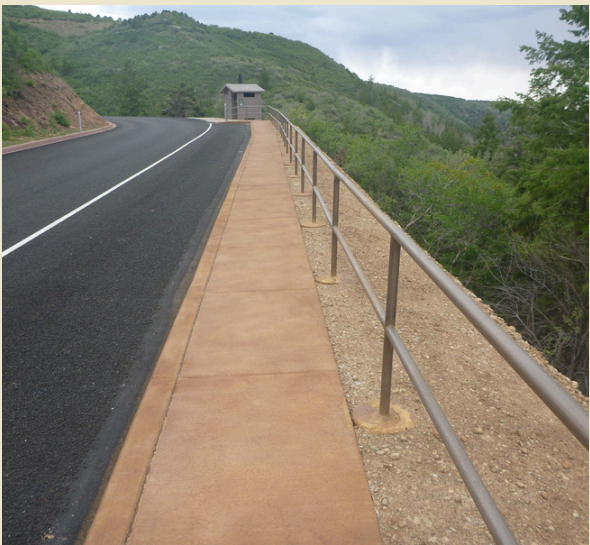
Natina-treated rail and walkway
